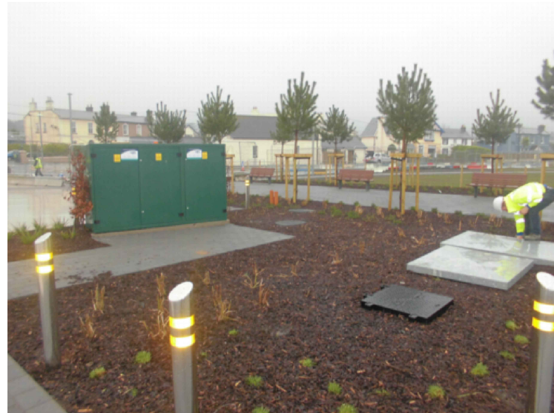
IMAGE 001 - FOUL PUMPING STATION EXAMPLE
